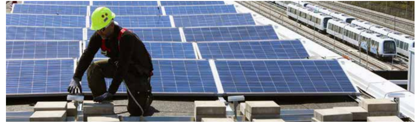
In 2016, the Control and Maintenance Centre in Vasbygade was equipped with solar panels.
